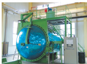
浇注罐 Casting tank
