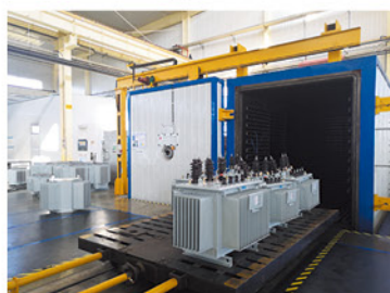
干燥罐 Drying tank
