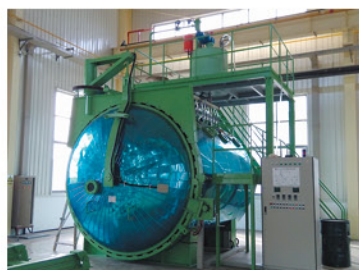
浇注罐 Casting tank
