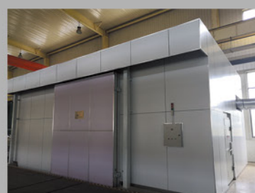
局部放电及噪音屏蔽实验室 Partial discharge and noise shielding laboratory
