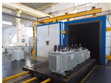
干燥罐 Drying tank
